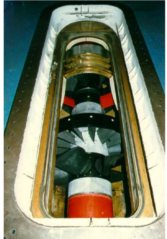
High Reynolds Number Pump Test Facility Installed in the GTWT Test Section
